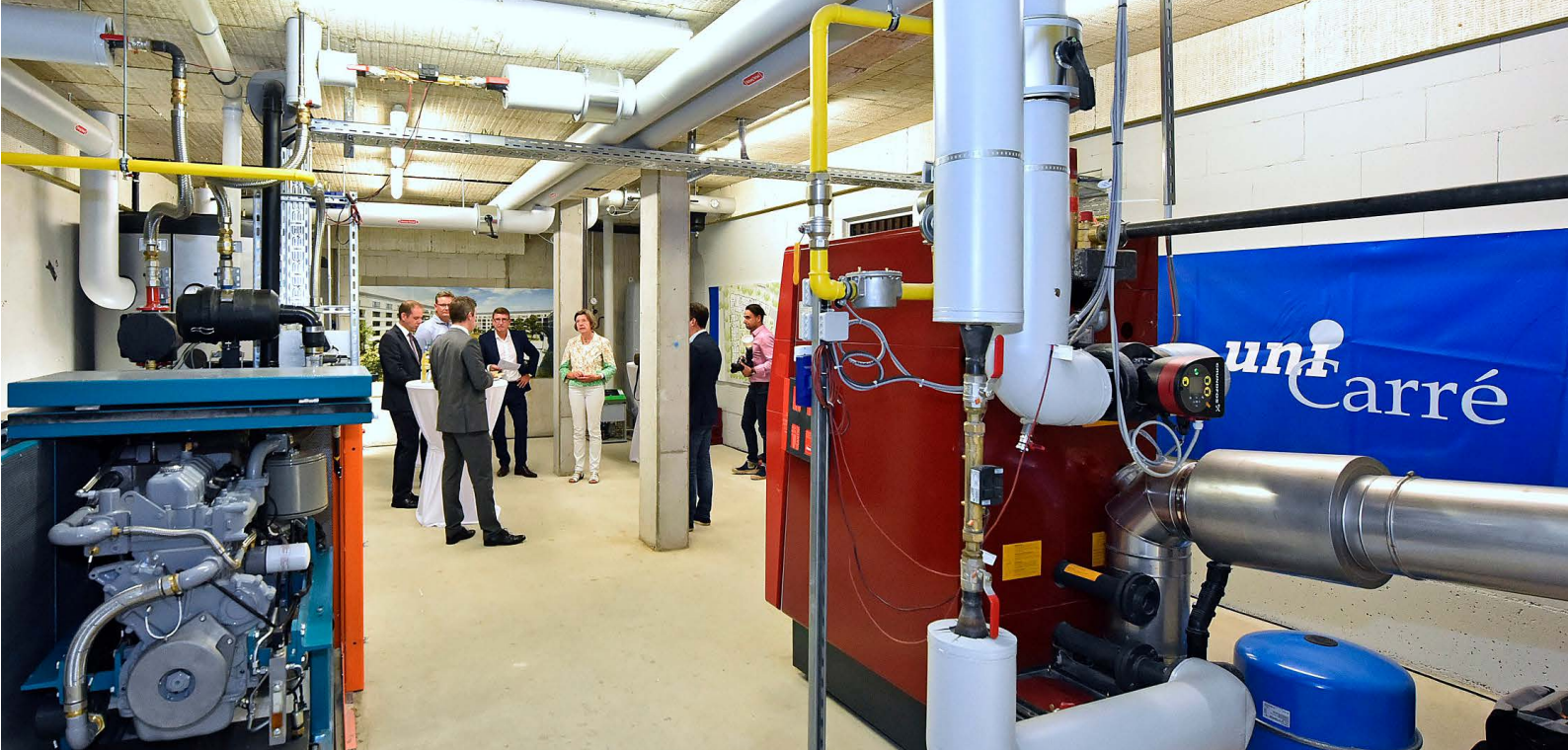
Combined heat and power plant in the Uni-Carré
