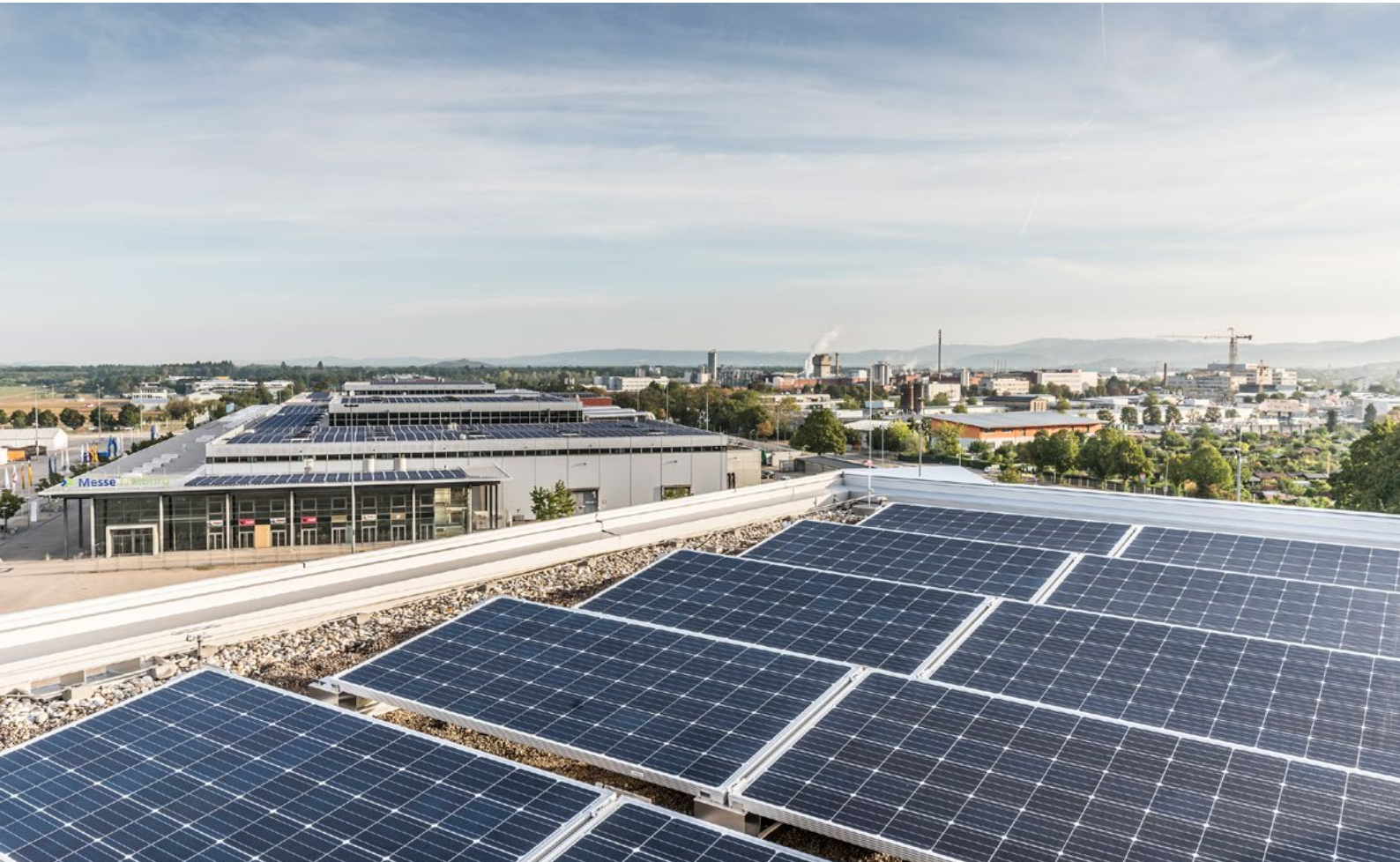
Photo 17: The roof of the trade fair building covered with photovoltaics and a view over the North Industrial Park. © FWTM, Spiegelhalter
